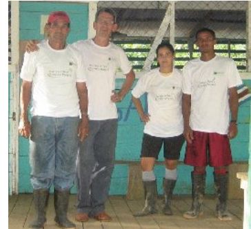
Our partner's team performing repairs at a local school in Costa Rica
